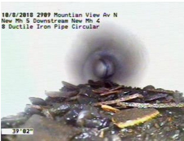
Figure 6.2-2 Debris and Sediment, Some of which Appears to be Chunks of Cement Mortar Lining Material
