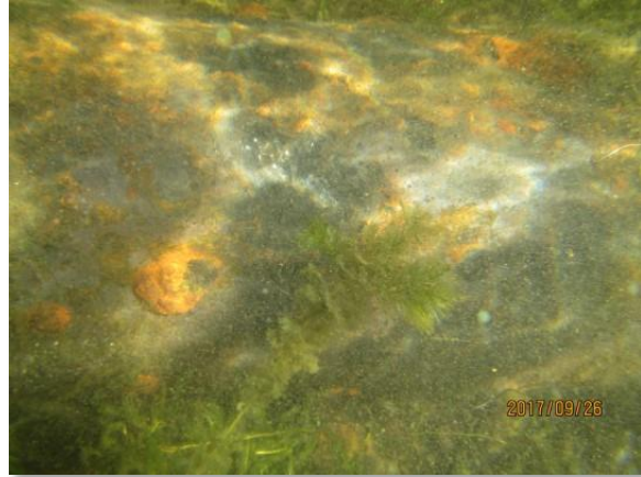
Photo C-30. Corrosion tubercles underneath dirt/debris layer
