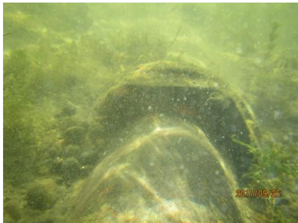
Photo C-27. Mechanical joint at fitting
