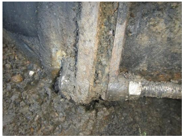
Photo C-8. Stainless steel bolts on mechanical joint
