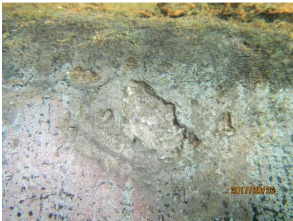
Photo C-21. Pitted surface; up to 0.06-inch-deep pits; dimple pattern (DIP)
