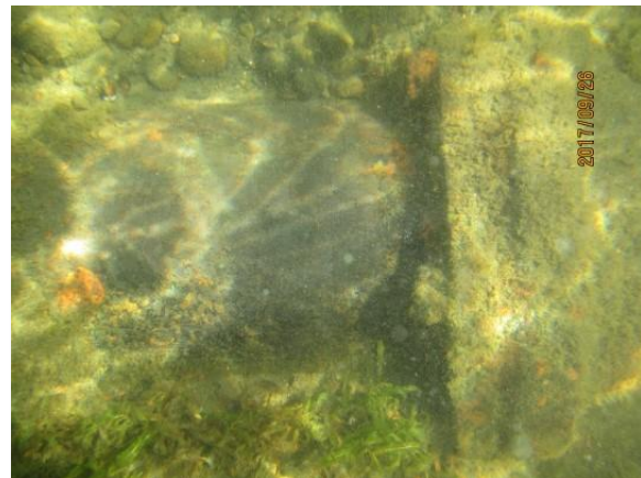
Photo C-28. Top view of mechanical joint
