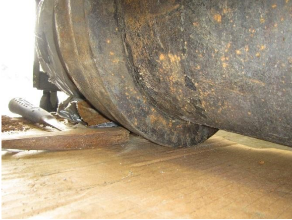
Figure 6.3-6 Exterior Surface of Manhole 5 Sample with Scattered Minor Pitting
