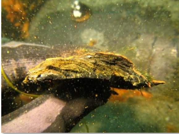
Photo C-62. Scale/tuberculation removed from pipe surface
