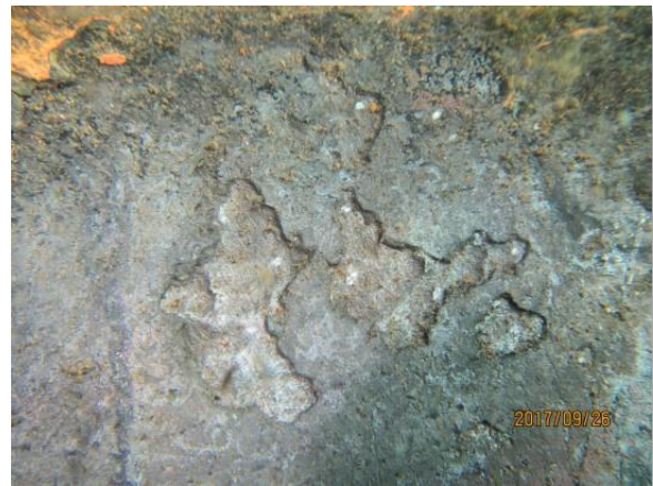
Photo C-22. Pitted surface; up to 0.06-inch-deep pits
