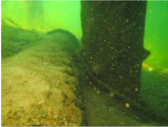
Photo 2-11. Lakeline sits only inches from dock piling near 3719 and 3805 Lake Washington Blvd. North
