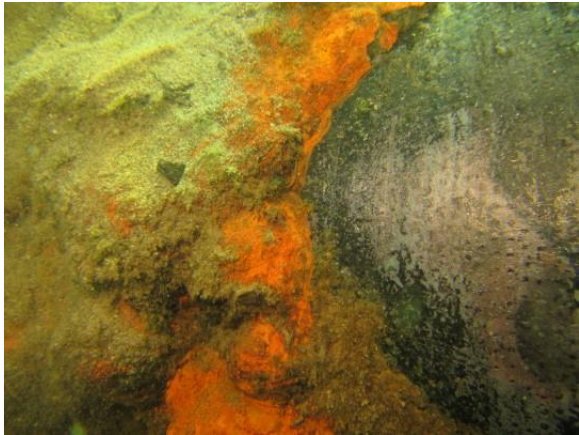
Photo C-64. Corrosion scale/tuberculation; dimple pattern on pipe surface (DIP)
