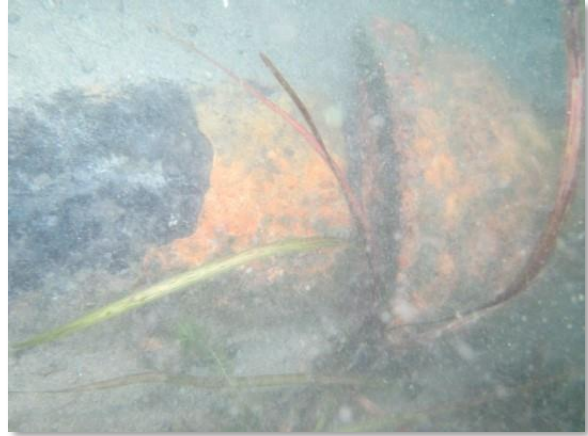
Photo C-38. Corrosion scale/tuberculation on bell/spigot joint
