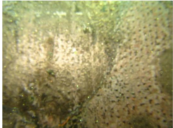
Photo C-65. Dimple pattern on pipe surface (DIP)
