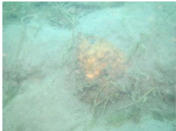
Photo C-55. Corrosion scale/tuberculation underneath dirt/debris
