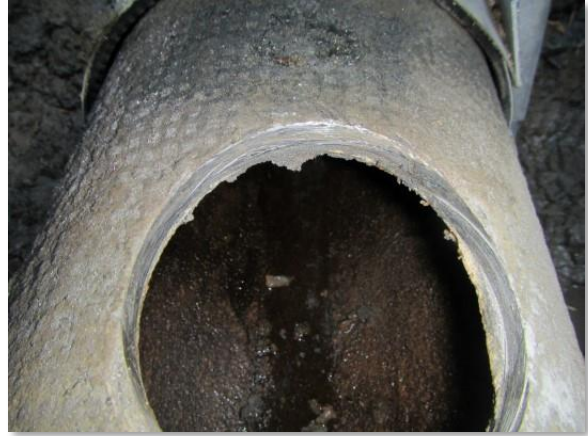
Photo C-10. Pipe coupon hole
