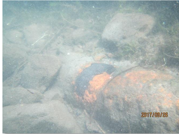
Photo 2-2. Area of scaling and tuberculation on mainline; large rocks around mainline at 2811 Mountain View Ave. North
