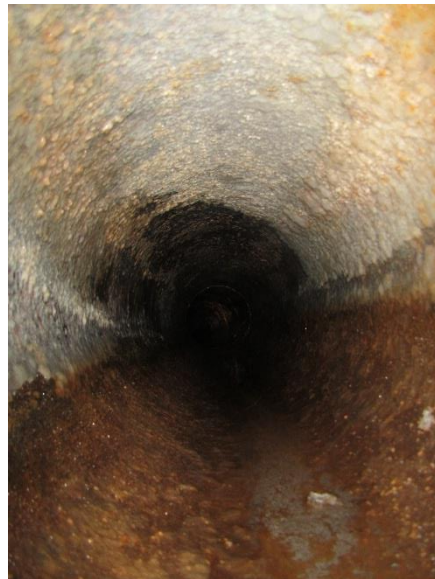
Photo 2-19. Interior of Lakeline looking downstream; appears to be corrosion staining on lower half of pipe
