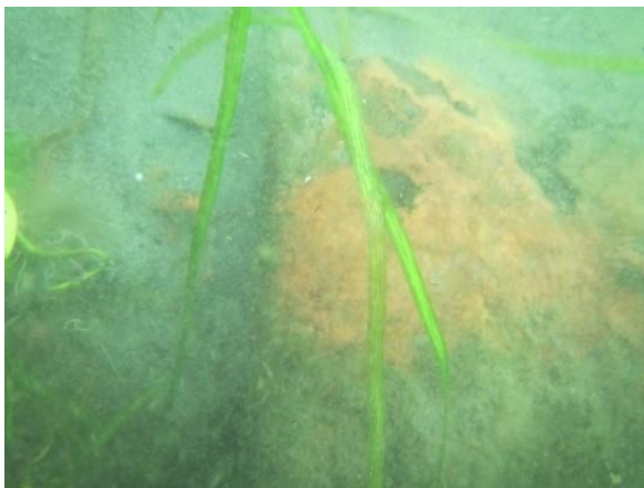
Photo C-33. Corrosion scale/tuberculation on bell portion of push-on joint
