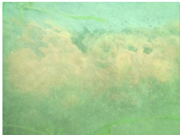
Photo C-34. Corrosion scale/tuberculation on individual pipe segments
