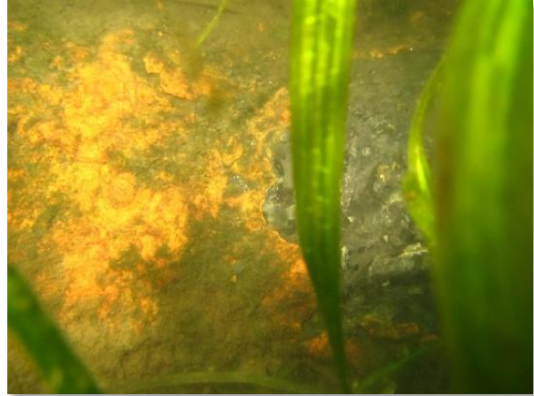
Photo C-71. Corrosion scale/tuberculation on pipe
