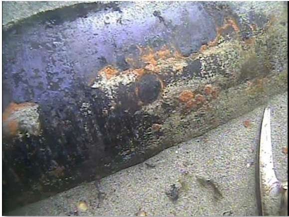
Photo 2-1. As-found condition of mainline with minor corrosion tubercles
