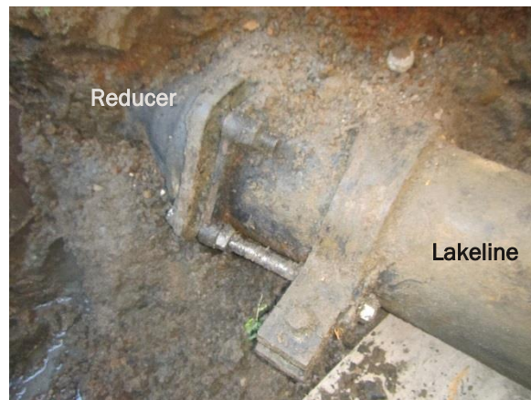
Photo 2-15. 4x8-inch reducer and restrained joint in good condition
