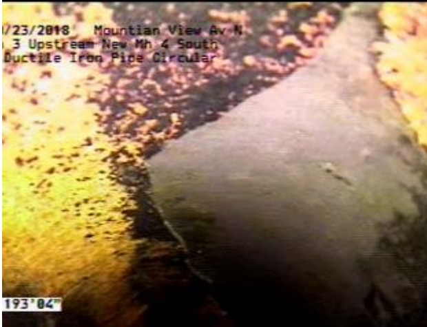
Figure 6.2-1 Typical Lining Delamination with Smooth Metal Surface Behind
