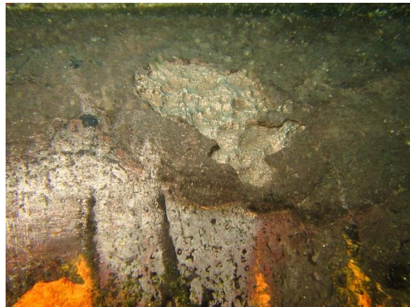
Photo 2-4. Moderate pitting and graphitized layer after wire-brushing surface
