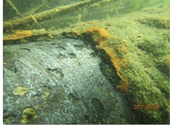
Photo C-18. Pitting up to 0.06 inches deep; scale/deposits on pipe exterior
