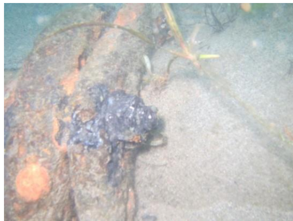
Photo C-48. Nuts, bolts glands of mechanical joints with corrosion but in fair condition
