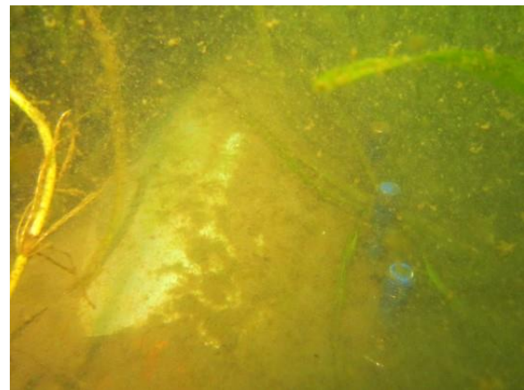
Photo C-73. 2-foot long repair clamp; appears to be a stainless steel clamp with coated bolts
