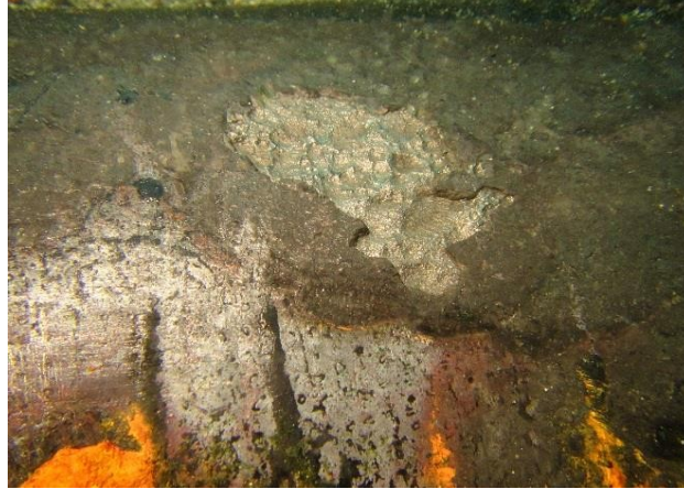
Figure 6.1-4 Moderate Pitting and Graphitized Layer After Wire-Brushing Surface
