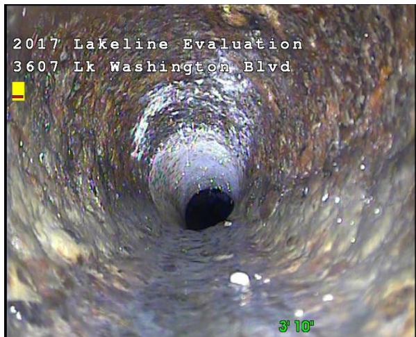
Photo 2-24. Staining on lateral interior
