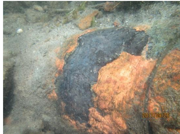
Photo C-16. Close-up of corrosion scale/tuberculation on pipe
