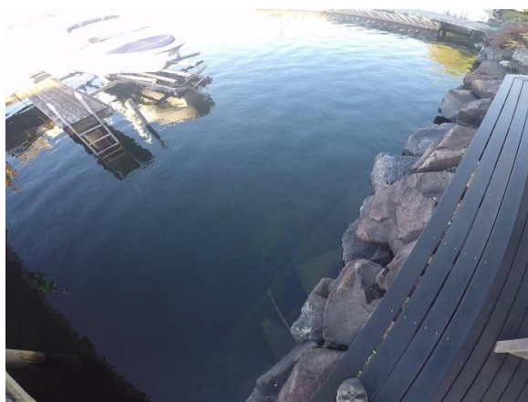
Photo 2-9. Rip-rap directly adjacent to and above Lakeline at 2811 Mountain View Ave. North
