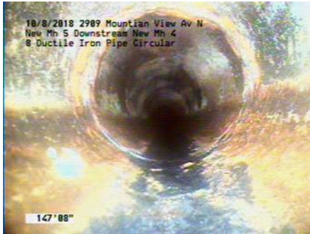
Photo 3-17. Typical corrosion deposits at joint.
