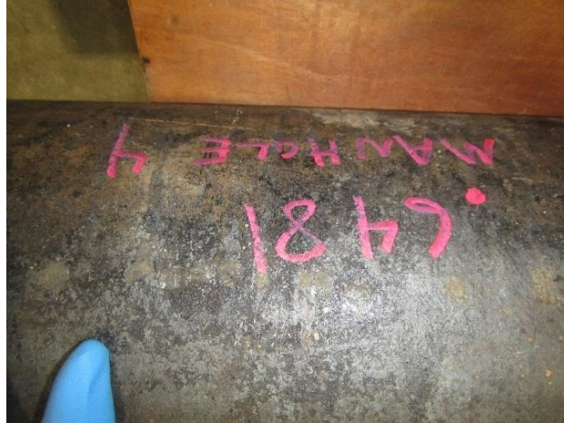
Figure 6.3-3 Exterior Surface of Manhole 4 Sample with a Few Scattered Minor Pits
