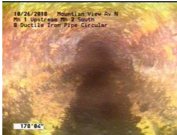
Figure 6.2-4 Typical Moderate to Significant Corrosion at High Points (Brown Area)
