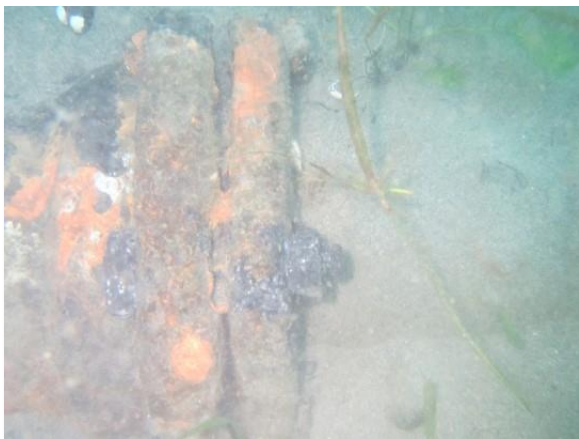
Photo C-47. Nuts, bolts glands of mechanical joints with corrosion but in fair condition
