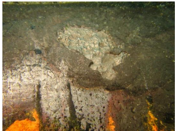
Photo C-59. Pipe and joint surface after removal of corrosion products; 0.125-inch-deep pit
