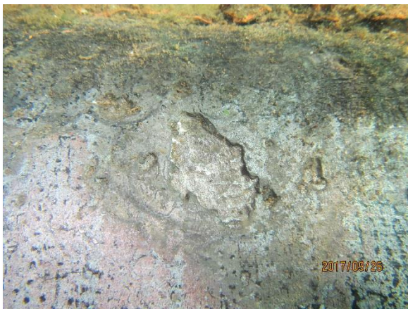
Photo 2-5. Pitting and graphitization
