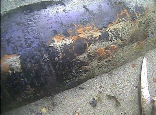
Figure 6.1-1 As-Found Condition of Mainline with Minor Corrosion Tubercles
