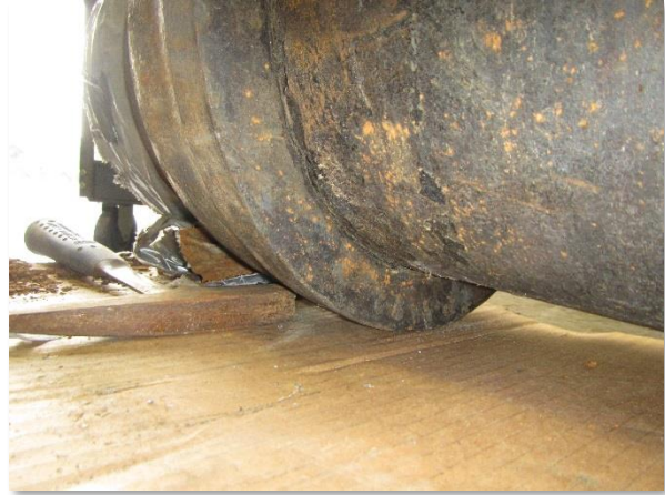
Photo 3-6. Exterior surface of Manhole 5 sample with scattered minor pitting.
