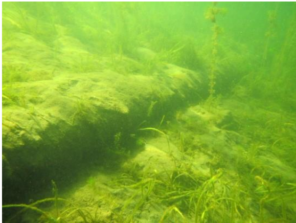
Photo C-66. Underside of pipe may not be fully supported
