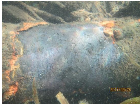
Photo C-20. Pipe surface underneath scale/deposits reach
