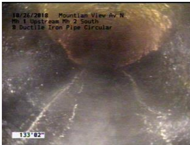
Photo 3-15. Typical moderate to significant corrosion at high point (brown area); black area appears to be stained mortar lining.
